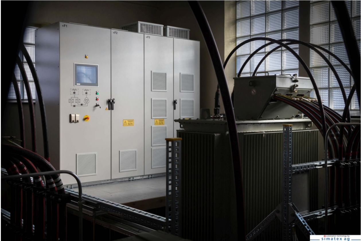
Inverted rectifier system of Simatex AG at "Wengen Rectifier"
